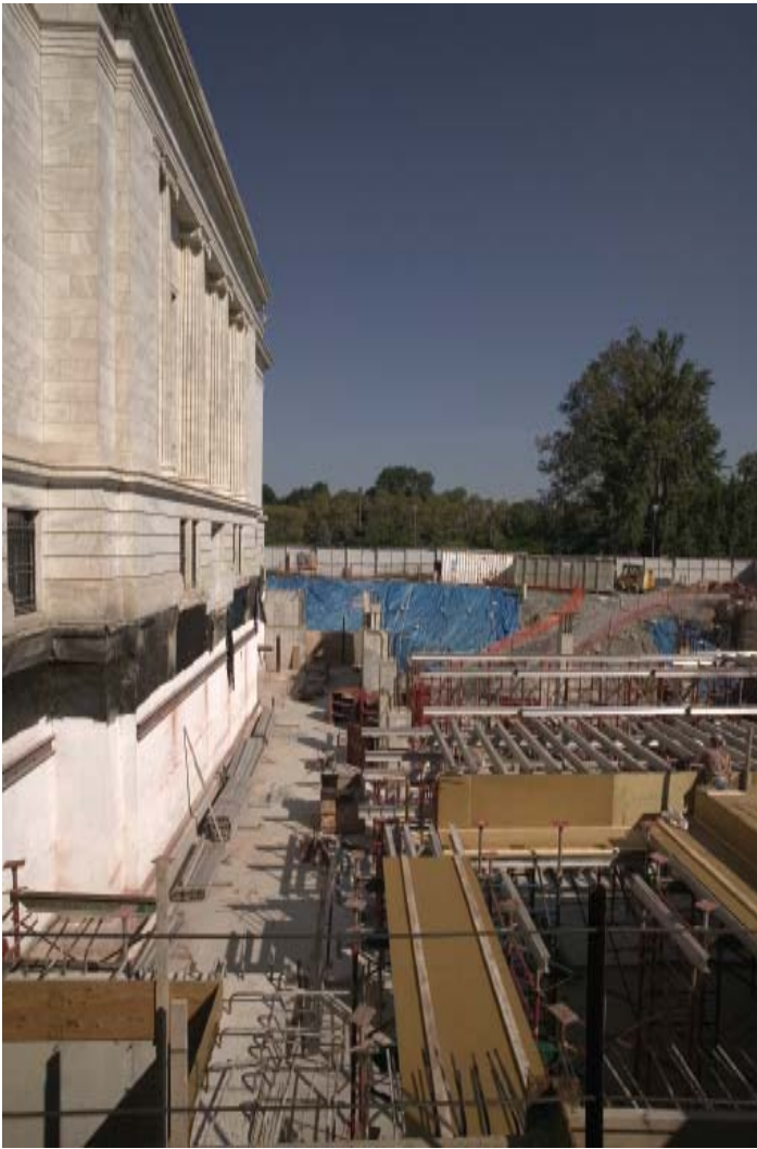
A major project to upgrade the museum's utility infrastructure took place on (and under) the east terrace.
